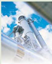
Stack gas analyzers
