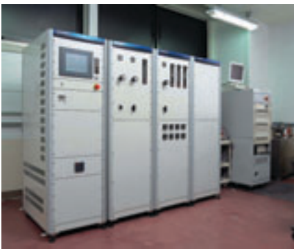
Fuel cell system evaluation laboratory in Head Office, Kyoto
